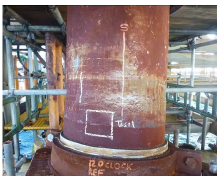
Corrosion location on Riser
